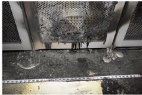
Figure A.1: Photograph taken during decommissioning of the ESS shows a pool of solidified aluminum on the floor in front of Rack 15 [1].
