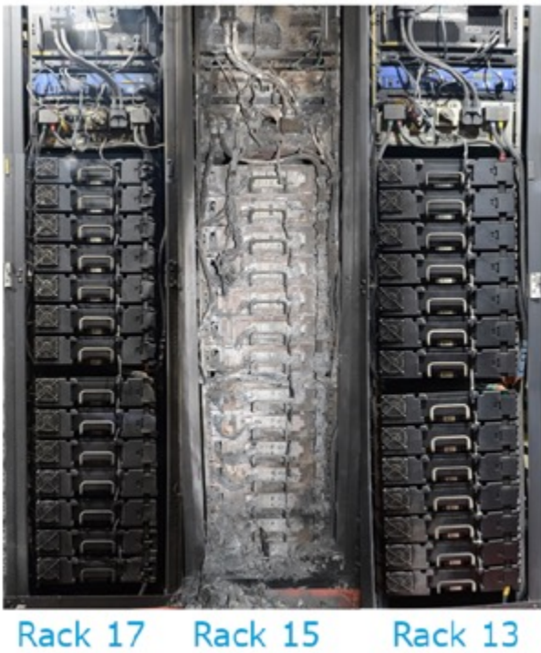
Figure 13: Destruction of Rack at McMicken.
