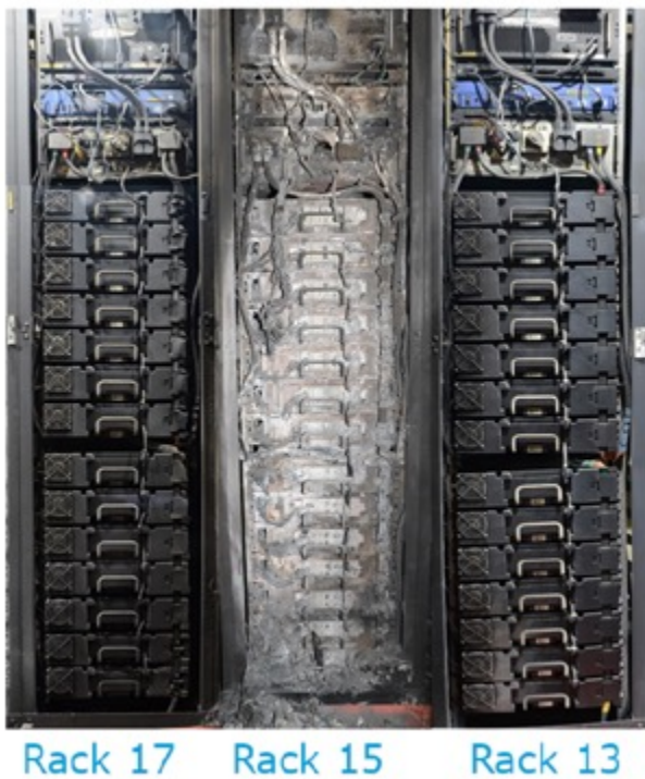
Figure 13: Destruction of Rack at McMicken.
